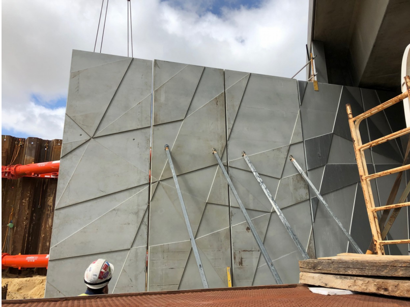
New abutments panels being installed next to existing panels for the bridge over Roe Highway
