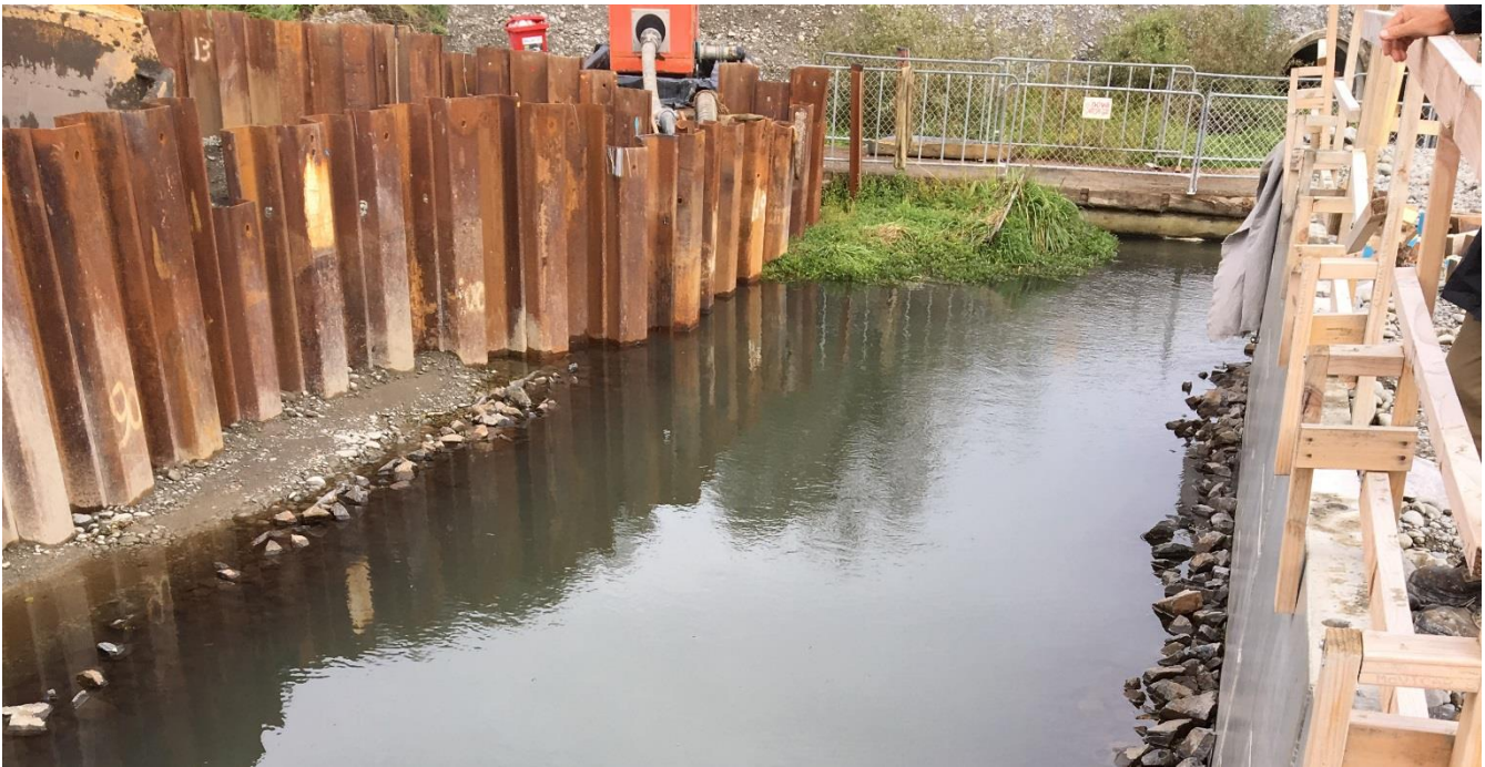
Above: Reinforced Earth® TerraClass® wall on north abutment with temporary sheetpiles on the south abutment.
