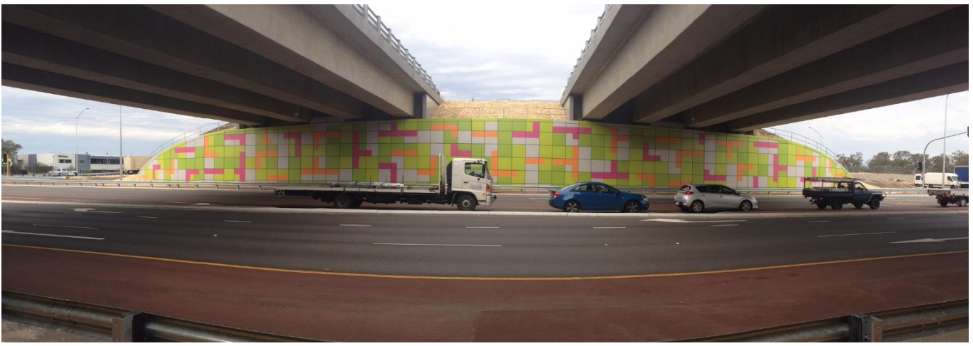
Above: Completed Reinforced Earth® Bridge Abutment at the Reid Hwy / Malaga Drive Interchange
