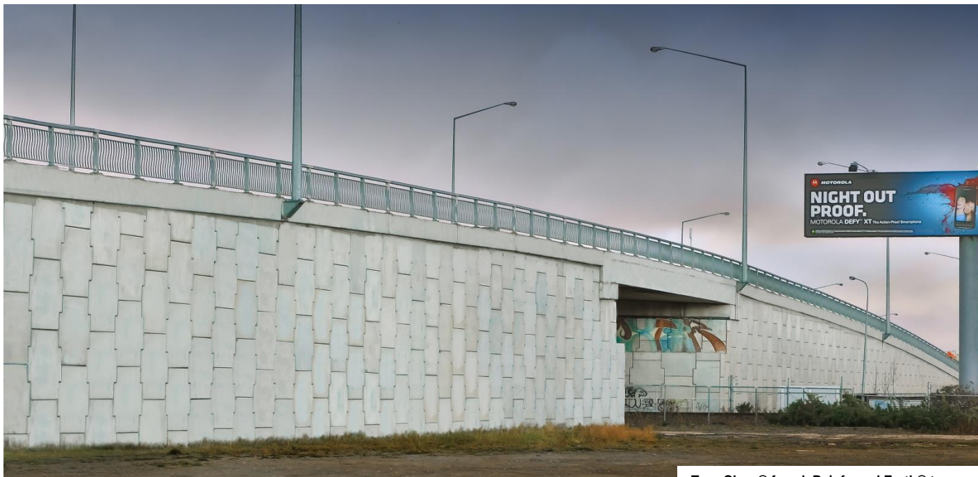
TerraClass® faced, Reinforced Earth® true abutment and retaining walls at Blenheim Rd Deviation
