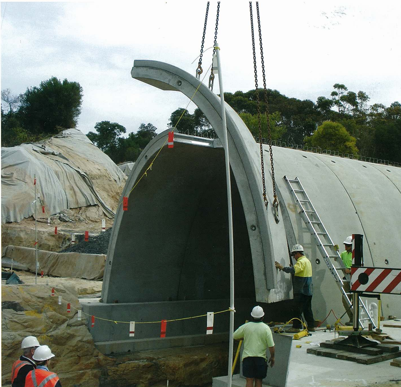
This large capacity precast culvert was recently installed at Leask Creek near Gosford on the NSW Central Coast.
