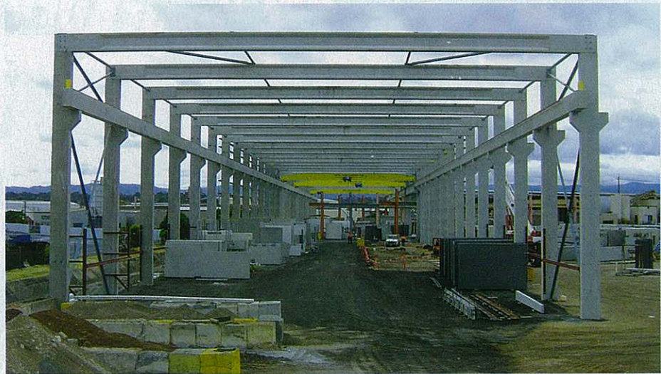
Adelaide precaster Bianco Precast built this 270m long portal frame building at its Gepps Cross manufacturing facility. The structure supports three 20t cranes.
