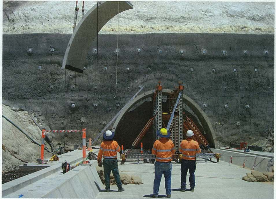
One of the arch units being installed at Rio Tinto's Kestrel coal mine in the Bowen Basin.
