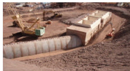
Main Picture: TechSpan® construction in the middle of a very congested, fully operational, Tom Price mine facility Top: Reclaim Tunnel Above: Escape Tunnel
