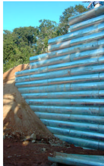
Main Picture: Sepon Copper – View of backfill, reinforcing straps, gravel drain behind structure, front face and panels ready for installation.
